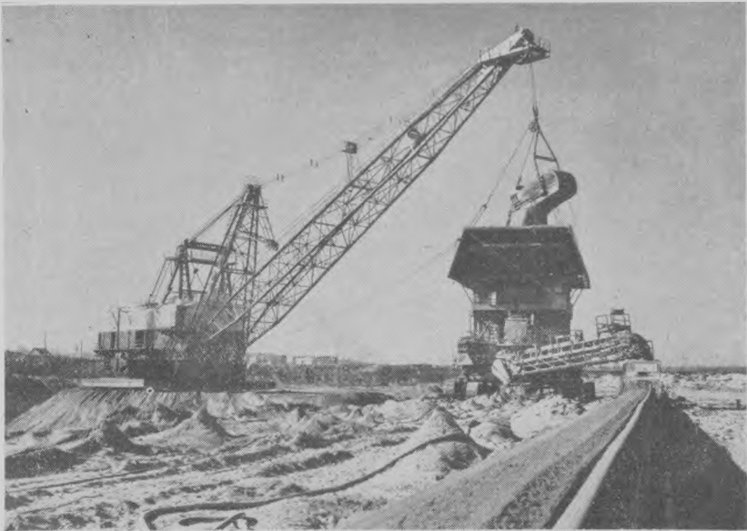
View of dragline and screening plant at the Morton mine. The model 1150-B dragline has a 180-ft. boom with a 30-cu. yd. bucket. The maximum digging depth is 110 ft. and the dumping height is 60 ft. Ground pressure of the base is 11 p.s.i. and of the walking shoes 21.9 p.s.i.
